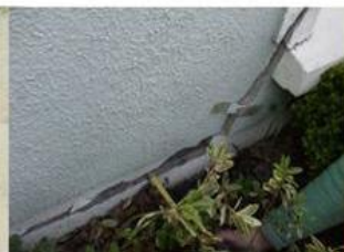
Damage Type 6 Lateral movement of external wall
