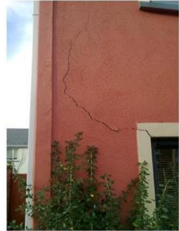
Damage Type 5 External wall cracking
