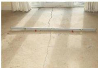
Damage Type 2 Lifting/Hogging of floor slab
