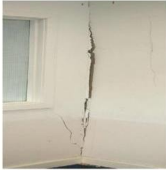
Damage Type 5 Bulging of wall finishes
