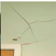
Damage Type 4 Cracking and Buckling of internal partition
