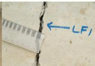
Damage Type 1 Cracking of floor slab
